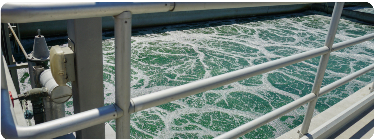
Aeration Basin at the Water Recycling Facility.
