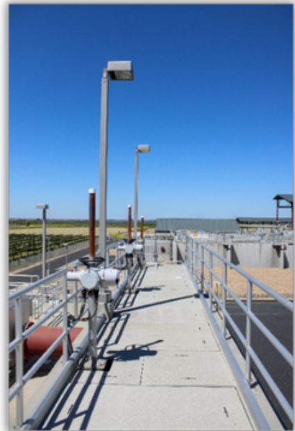
Light fixtures at the Water Recycling Facility.
