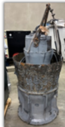
Sludge Pump before rehab.
