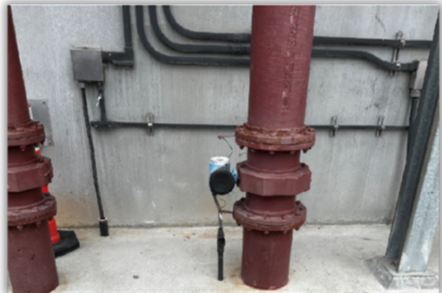
Influent pump station discharge piping.
