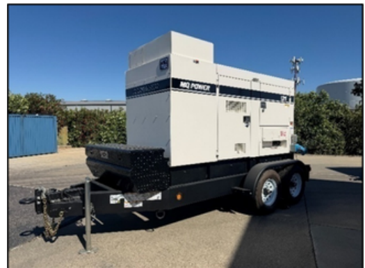
Generator used for emergency power outages.
