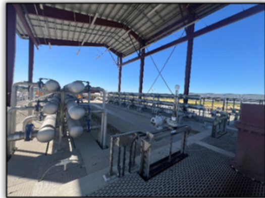
Membrane Bioreactor area.
