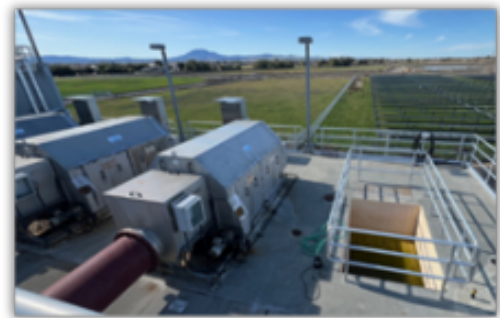
Water Recycling Facility Drum Screens.
