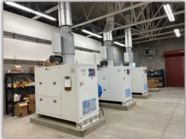
Aeration blowers for Membrane Bioreactor.
