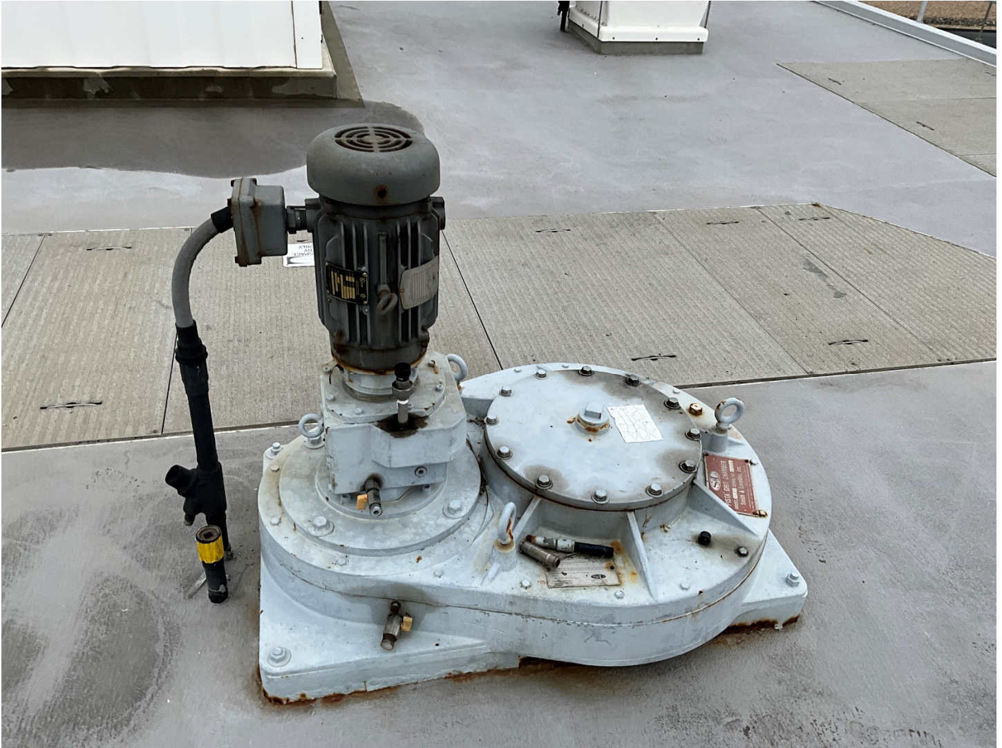
Corroded Vortex Grit Drive Gearbox and Motor
