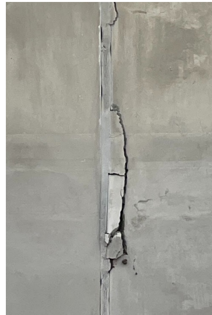
Photo 3 – Spalled concrete in sections of crack seen in photo 1
