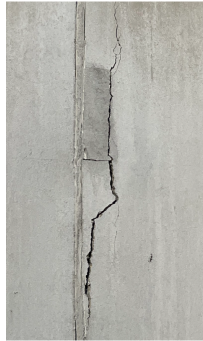
Photo 6 – Spalling at exterior face of south wall crack
