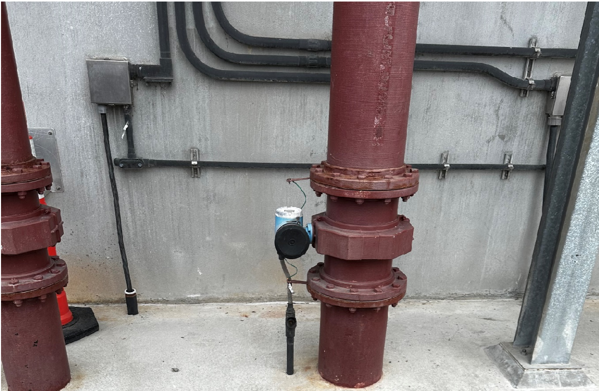
Beginnings of Coatings Failure on Above Grade Pipe
