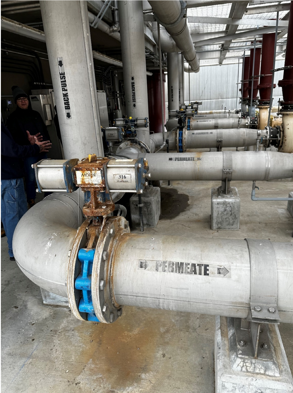
Figure 9.7. Permeate Valve and Actuator Corrosion
