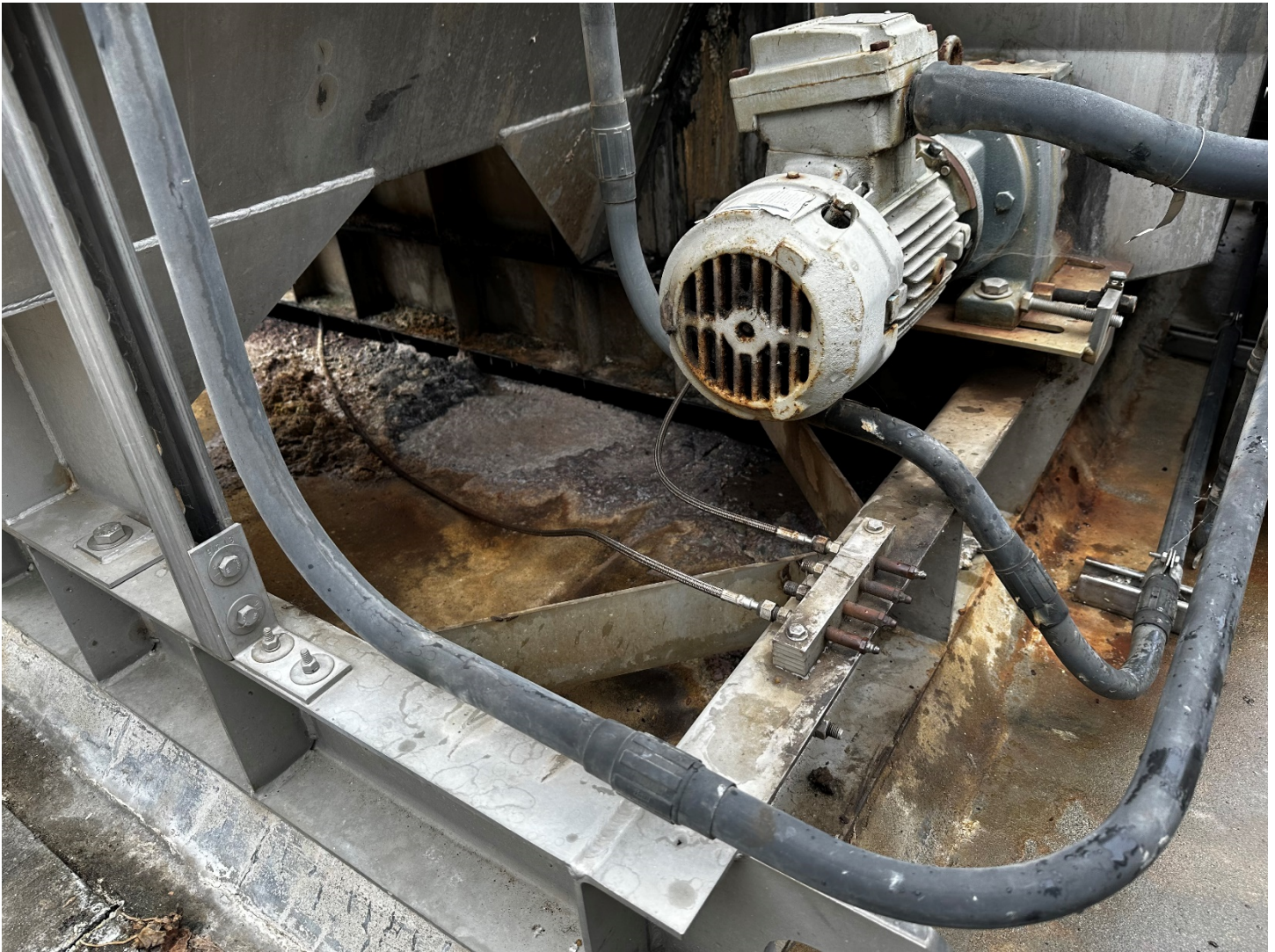
Concrete Corrosion Around Base of Drum Screens
