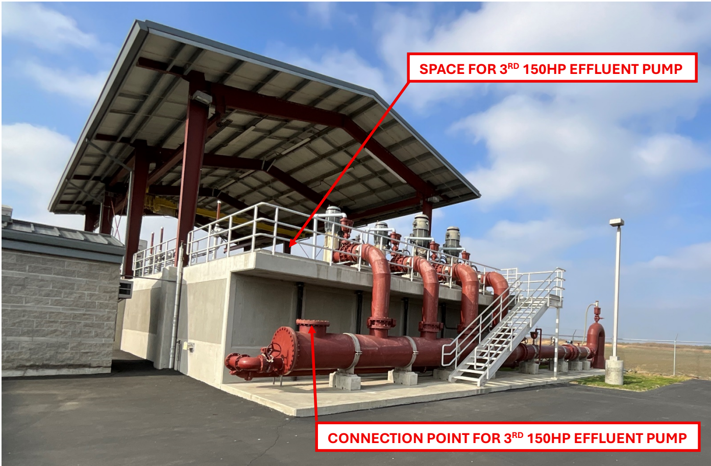
Location for 3 rd Large Effluent Pump
