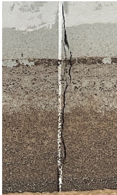
Photo 2 – Close up of crack in photo 1 depicting varying crack widths
