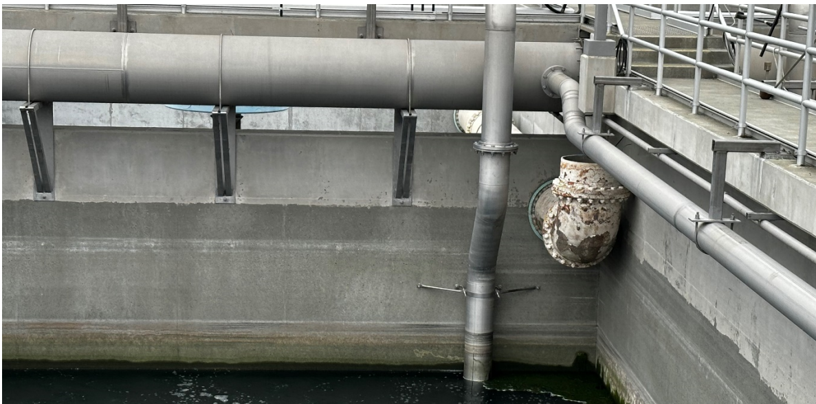
Figure 7.11. RAS Piping Coatings Failure
