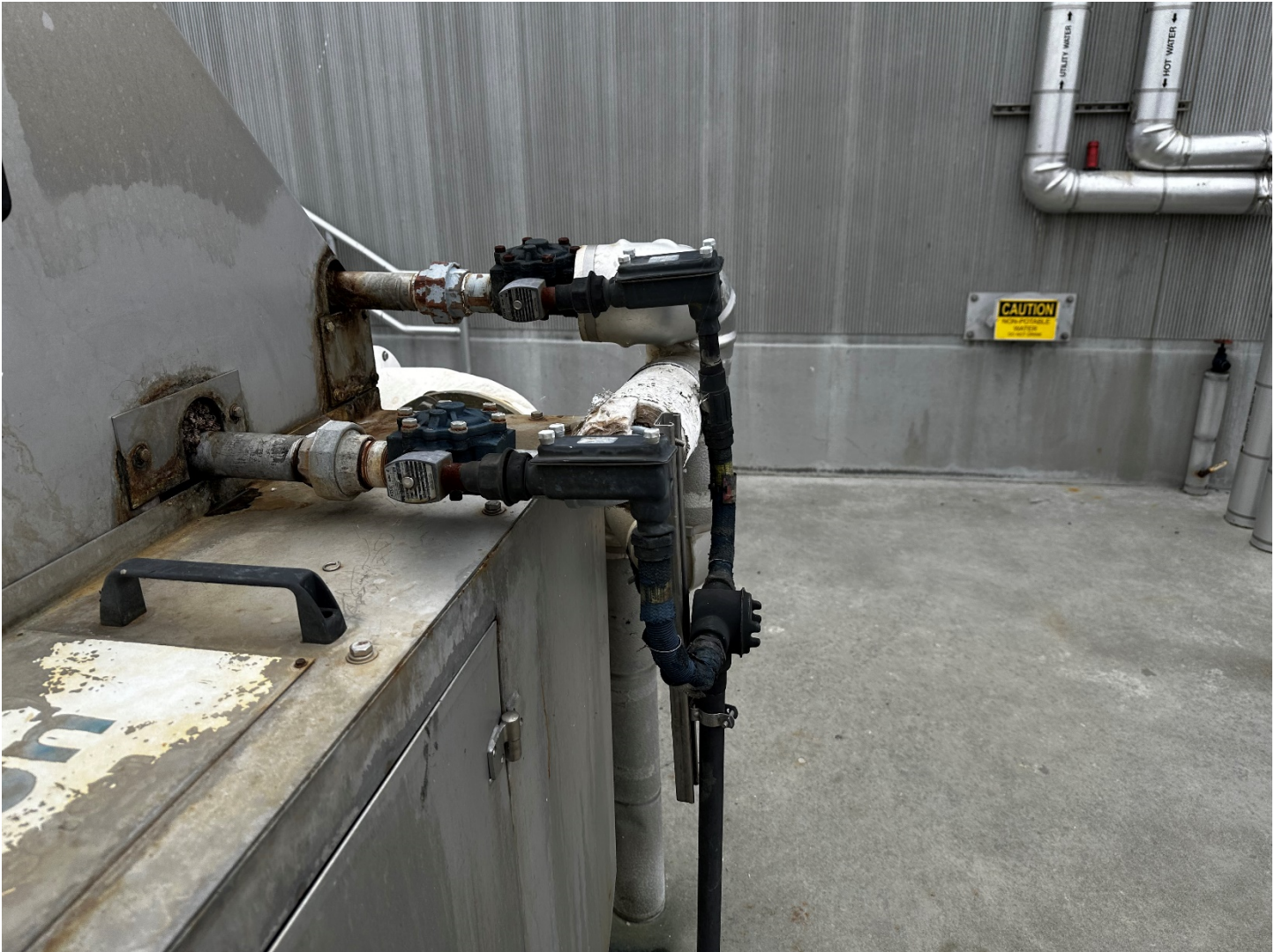
Corroded Utility Water Components
