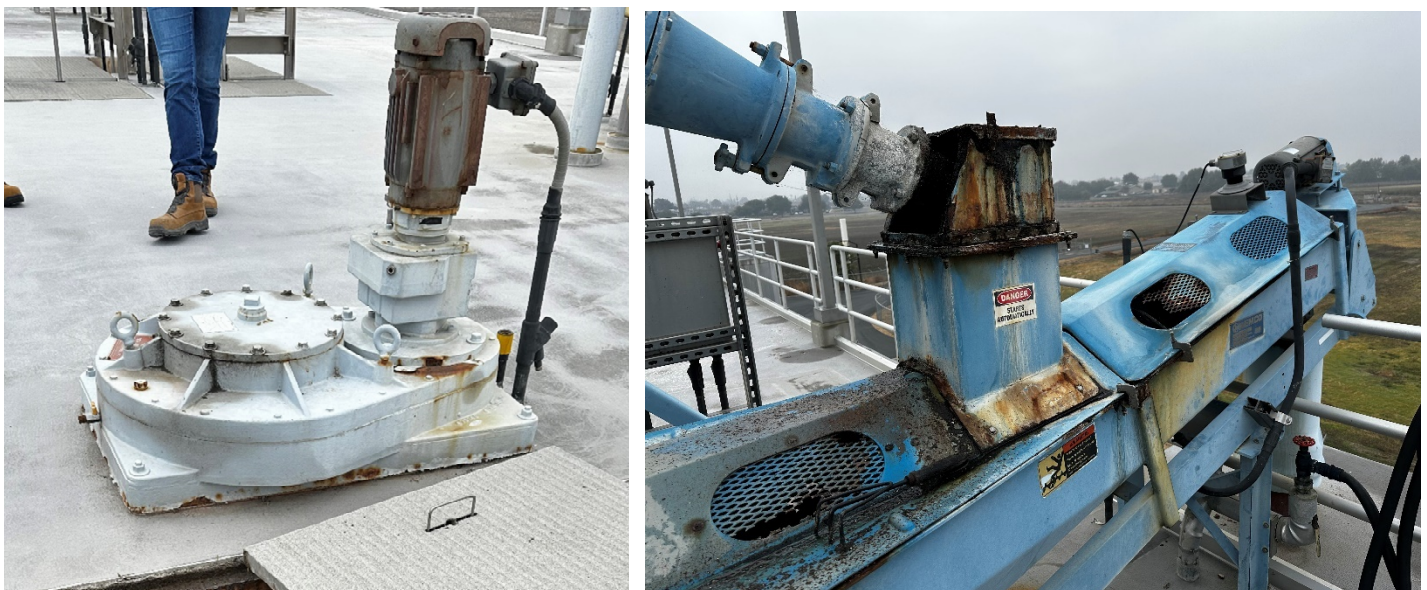
Figure 5.4. Grit Removal System Corrosion
