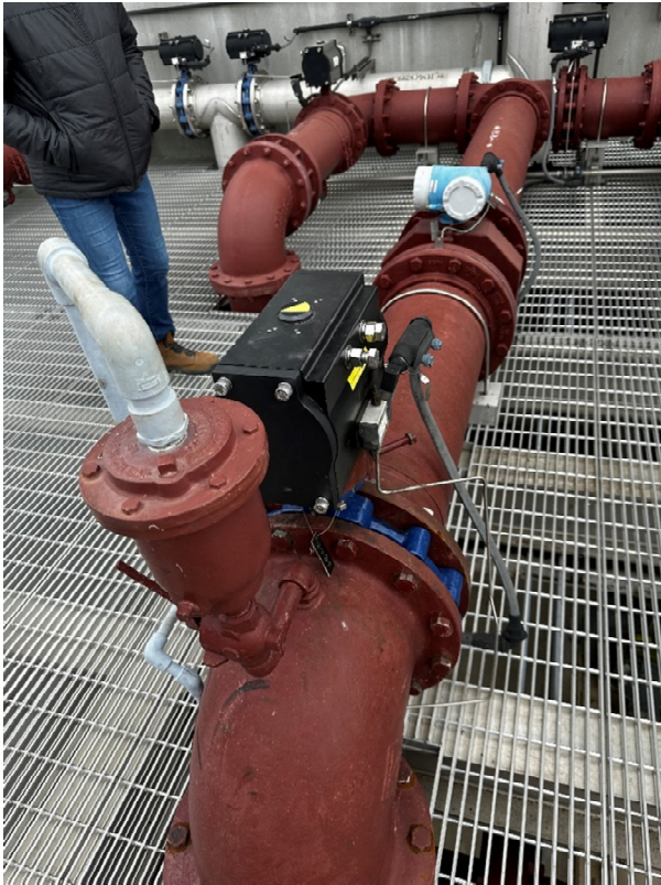
Figure 9.6. Permeate Flow Meter Isolation Valves
