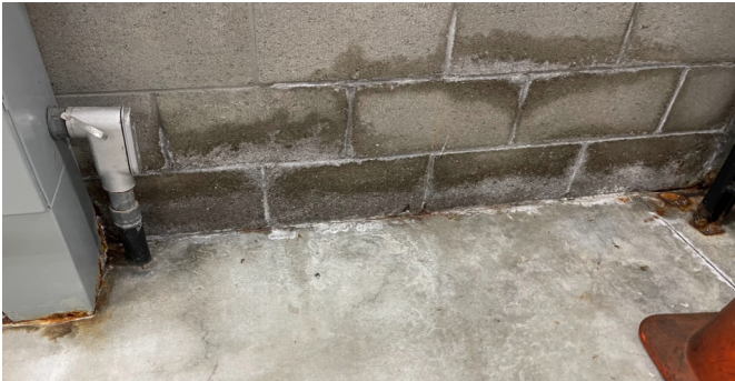
Photo 1. Damaged CMU wall at blower room due to H2S leakage.
