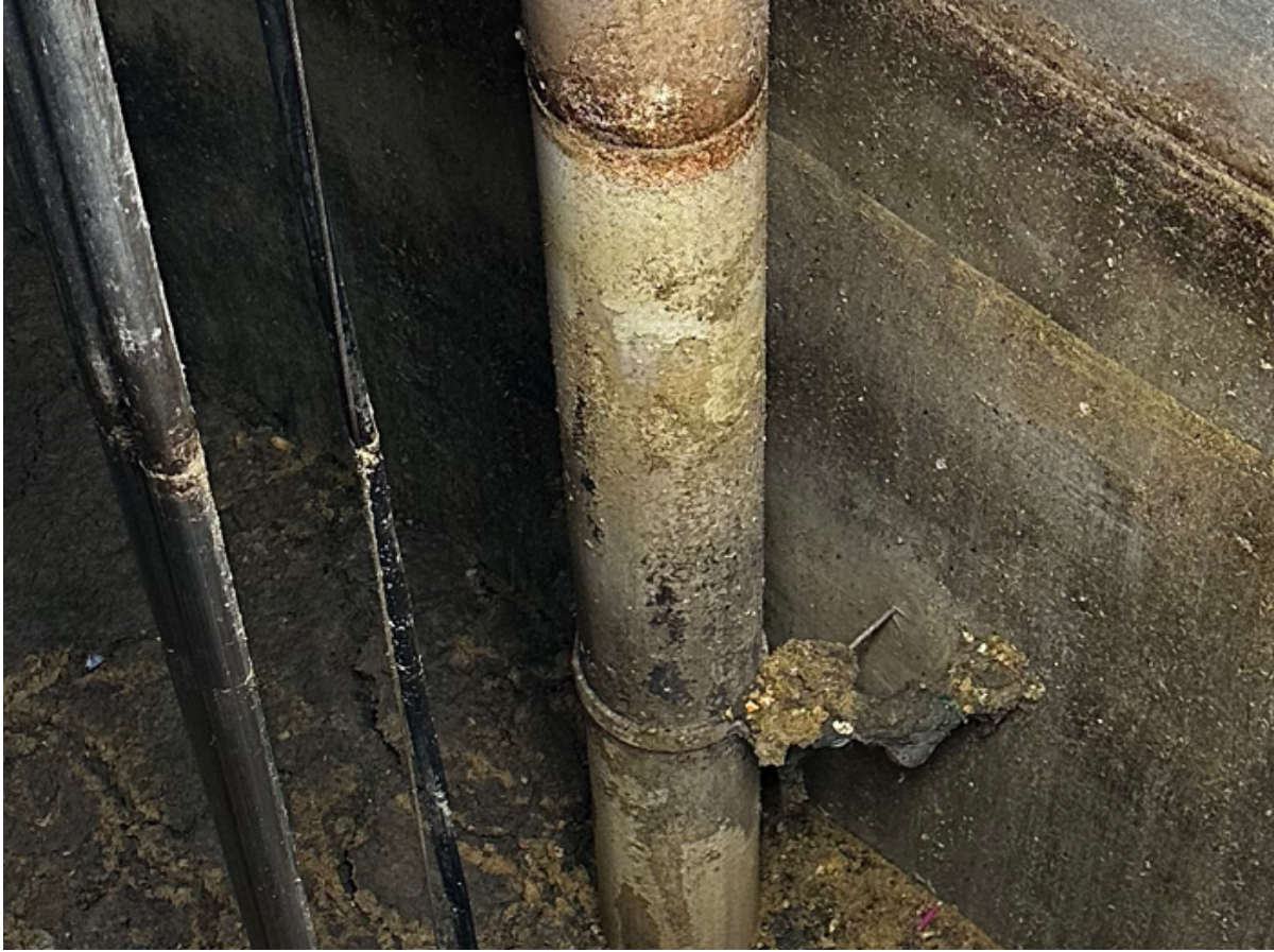
Corroded Piping in Wet Well with Coatings Failure
