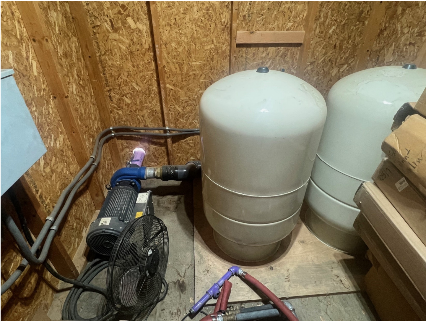
Existing Recycled Water Booster Pump and Hydropneumatic Tanks (existing pump to be removed, hydropneumatics tanks to remain)
