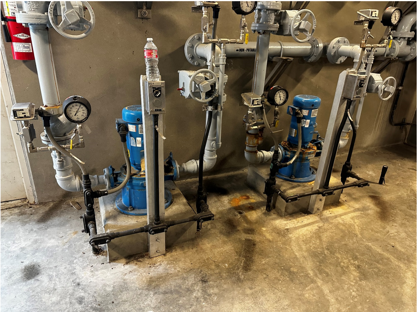
Existing (2) Washwater Booster Pumps With Space for Third
