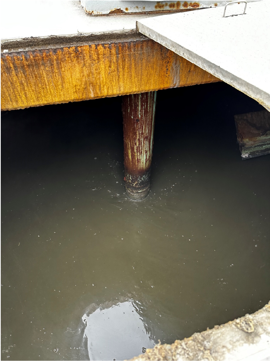
Corroded Vortex Grit Paddle Shaft
