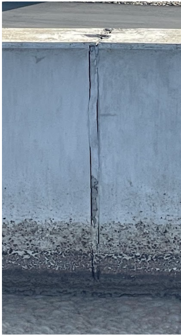
Photo 4 – Crack at interior face in south wall of aeration basin
