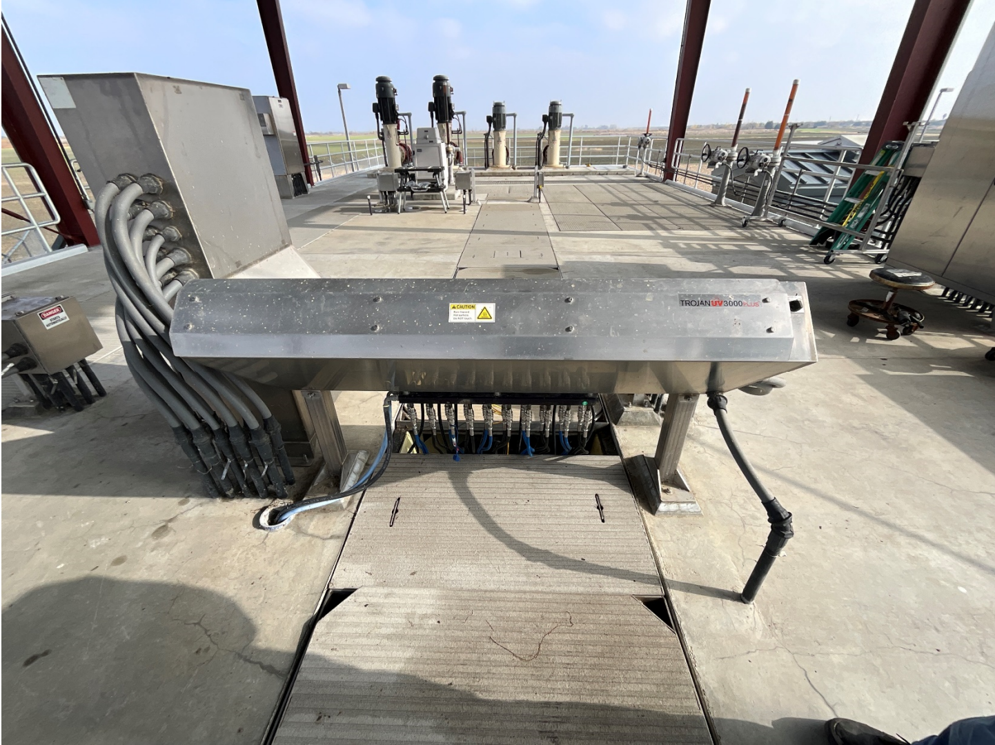
Existing Trojan UV System
