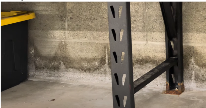
Photo 3. Damaged CMU blocks adjacent to area seen in photo 1.
