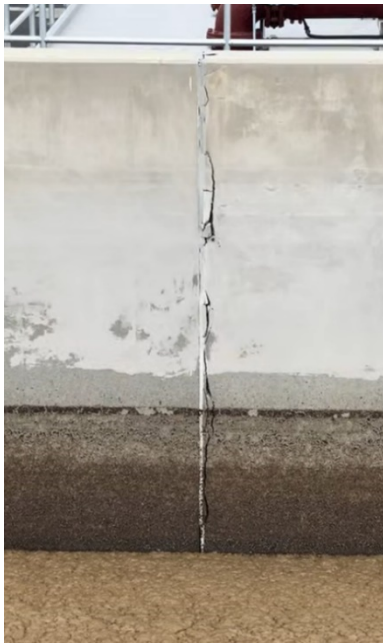
Photo 1 – Crack along CJ at north basin wall interior face
