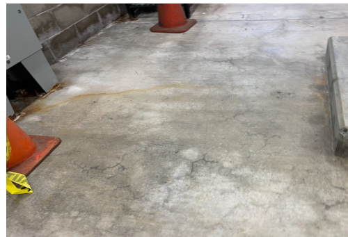
Photo 4. Minor damage to slab in area of leakage
