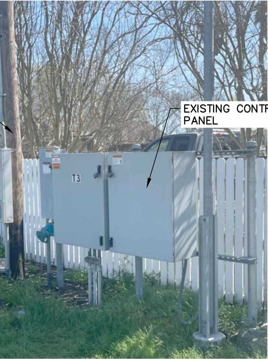
PHOTO 2 - CONTROL PANEL 2 NOT TO SCALE
