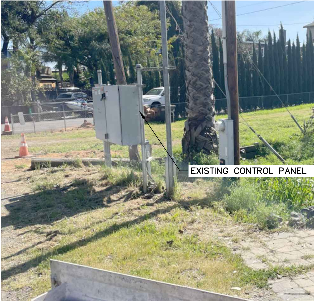
PHOTO 1 - CONTROL PANEL NOT TO SCALE
